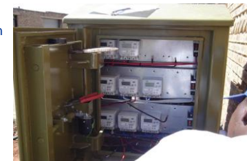
Up to 12 split meters in a Kiosk
