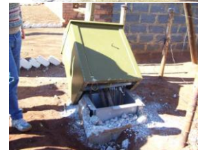
Attempted illegal connection -- failed
